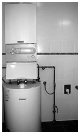
b) Gas Powered Water Heater with Tank
