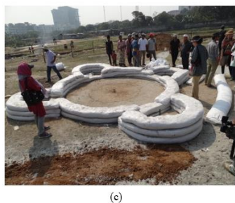
Figure 5: Step-3, 4, 5, 6: (a) Theoretical Base Plan. (b) Base making phase on the site adding sands (c) Base making progressive phase adding barbed wire with tamping earth bags.
