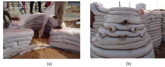
Figure 8: Step 9, 10: (a) Barbed wire in every rows of buttress walls used multipurpose (Kitchen, Toilet, Storage) (b) Buttress walls with ventilation and light with hollow plastics.
