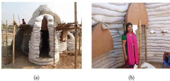
Figure 7: Step 8: (a) Doorway of dome on site (b) Inside of dome on site
